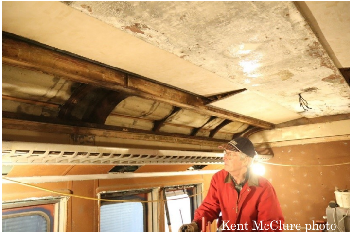
Bruce Backus is seen working on removing ceiling panels in the coach compartment of Wabash 1238.
