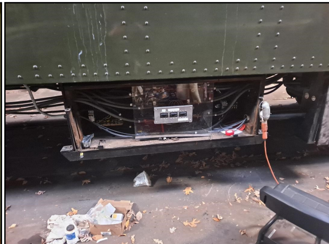
Left: New lights and heat controls are being installed in the light switch box.
