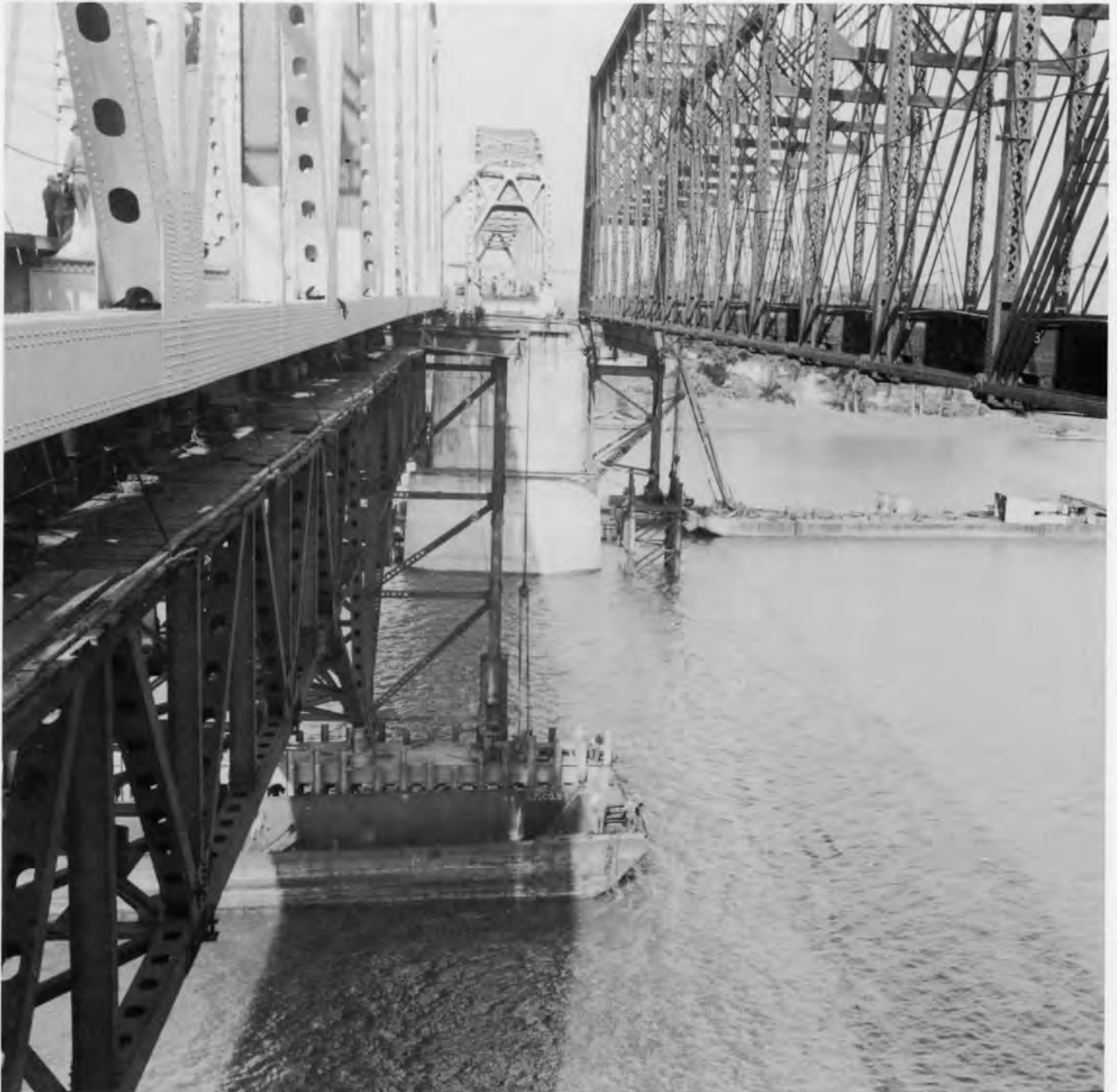
The old span has been moved to the side and the new span is being winched into position ICRR photo.
