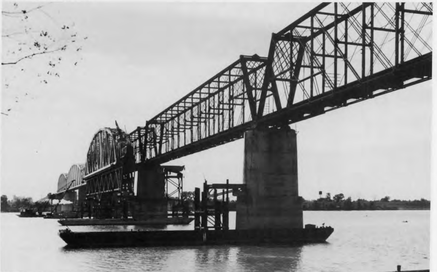
The fourth span of the new bridge is ready for placement in this photo.
