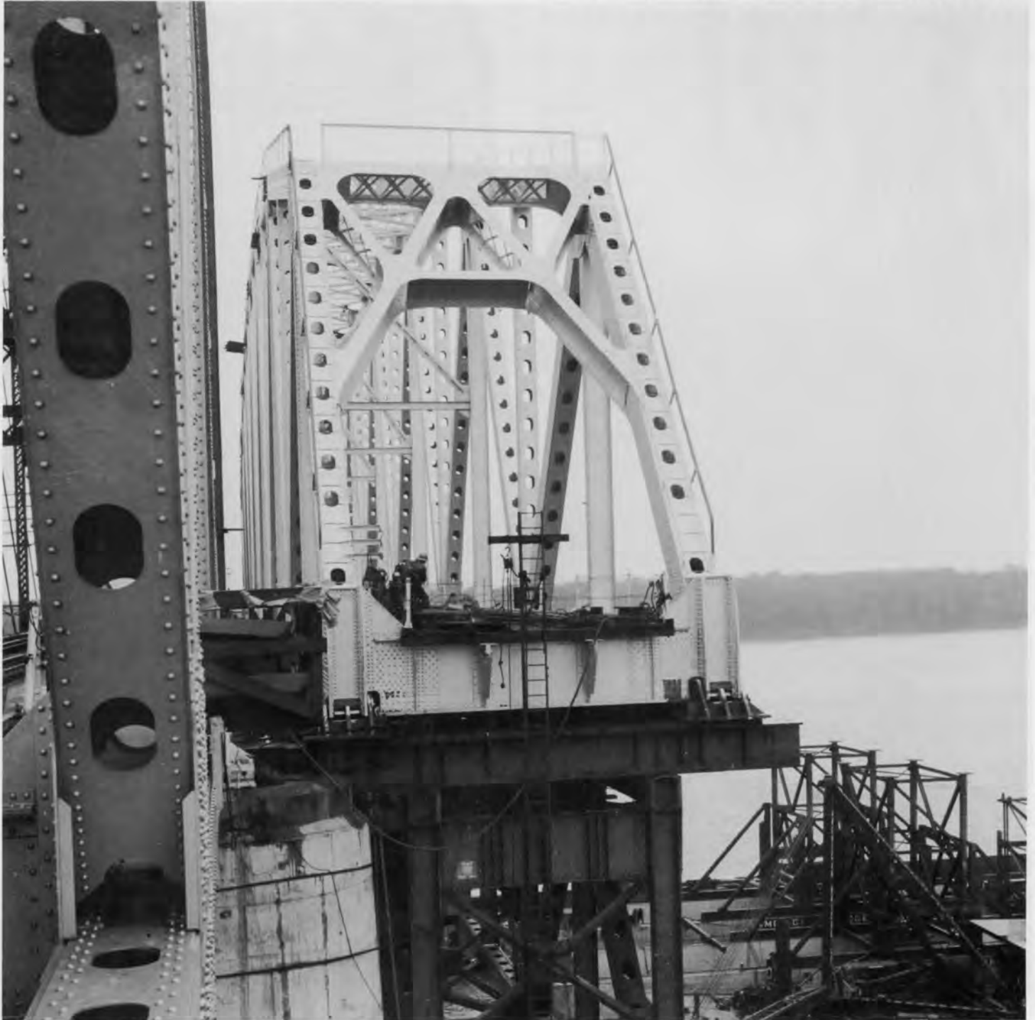
A completed new span is ready to be changed out with the old span.
