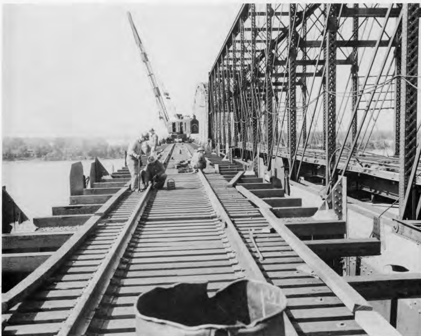
Rails are being secured to the deck of one of the new spans as it is built in place next to the old span that it will replace. ICRR photo.
