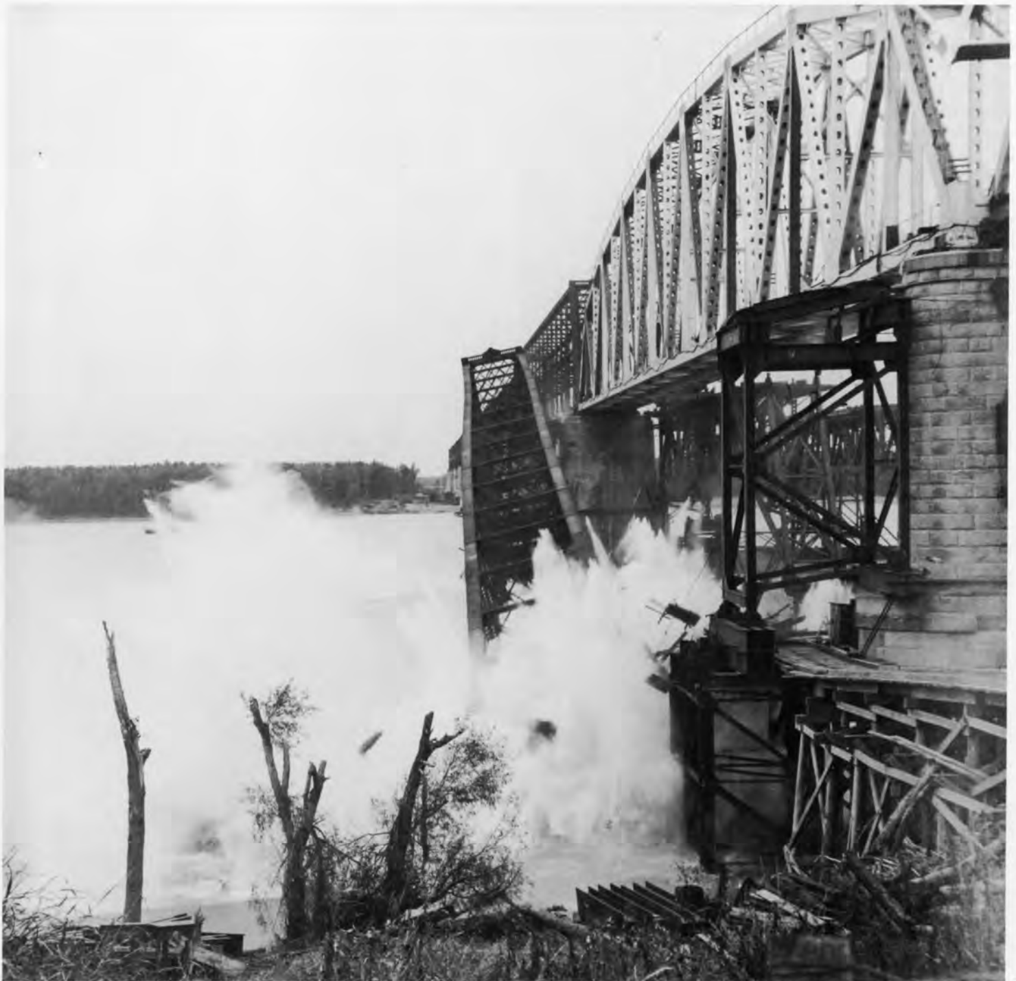
The first span of the old Cairo Bridge plunges into the Ohio River while the new replacement span sits in place and ready for traffic. ICRR photo.
