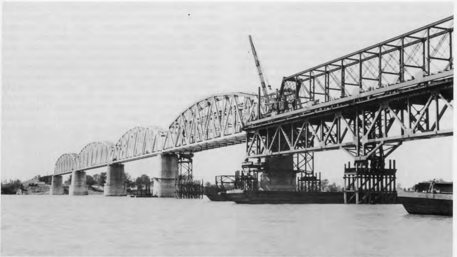
The new fourth span is in place while the old span still rests next to it. Some of the decking was removed before the old spans were slid into the river. In the meantime the 200' spans which were used to construct the larger spans upon, are in position and work is well underway on span #5. ICRR photo.
